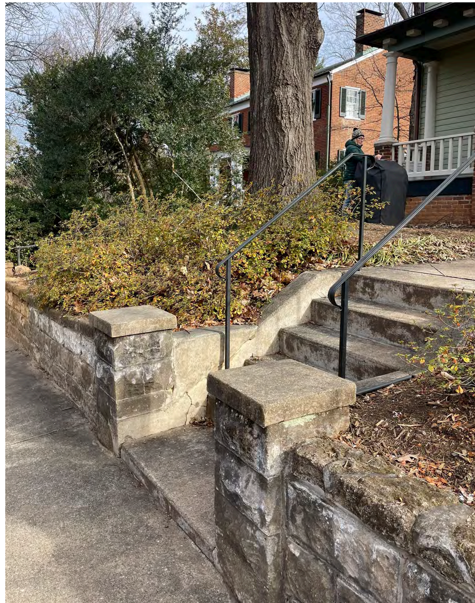
EXISTING WALL & COLUMNS TO REMAIN. NEW CHEEK WALL & STAIRS TO REPLACE EXISTING.
