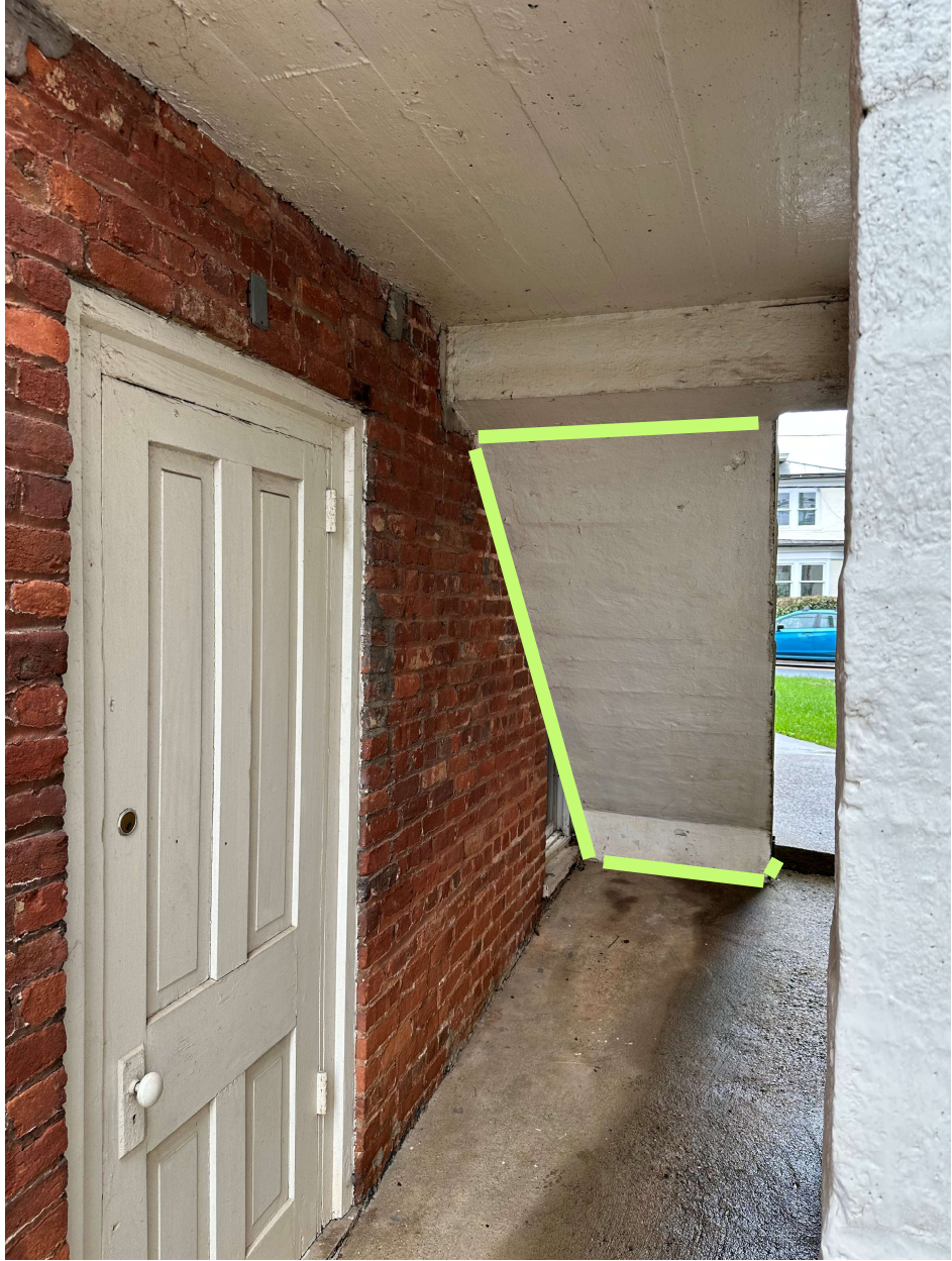
Attachment points to be repaired
