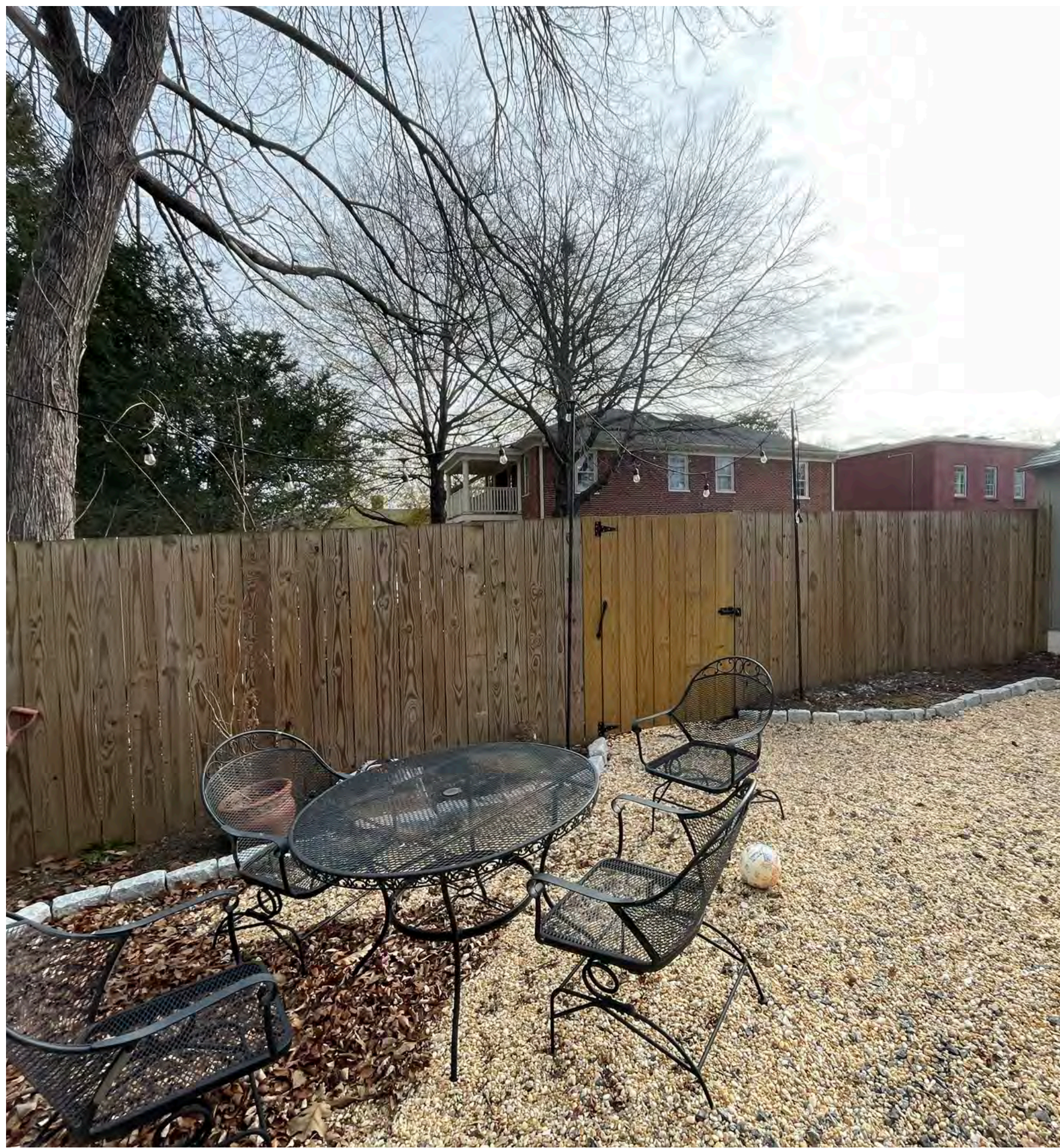
EXISTING PRIVACY FENCE FOR REPLACEMENT.
